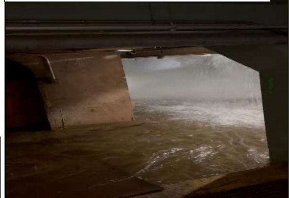
August 7, 2023 Main PS Catastrophic Valve Failure
